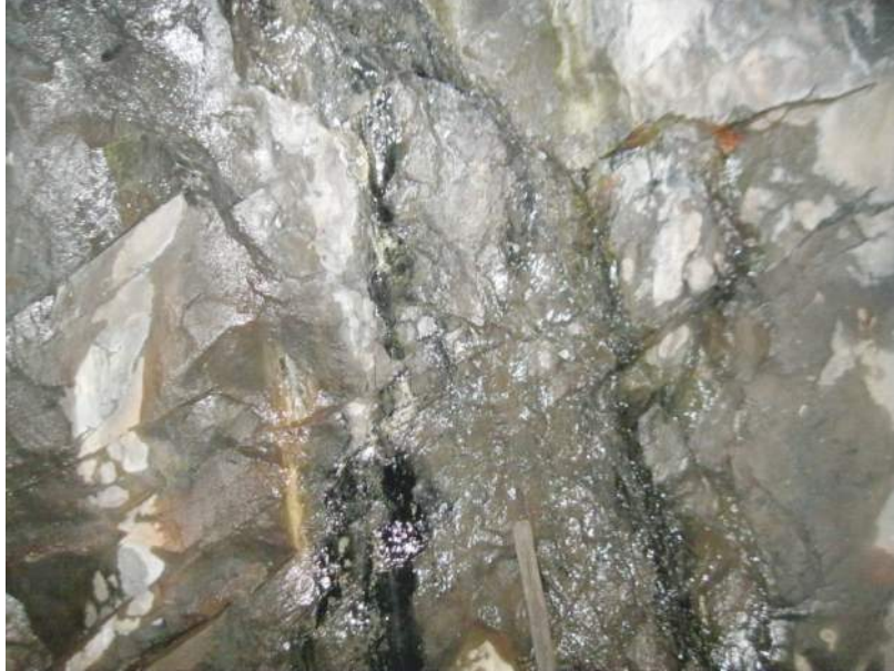
View of seepage in Tunnel No. 14
