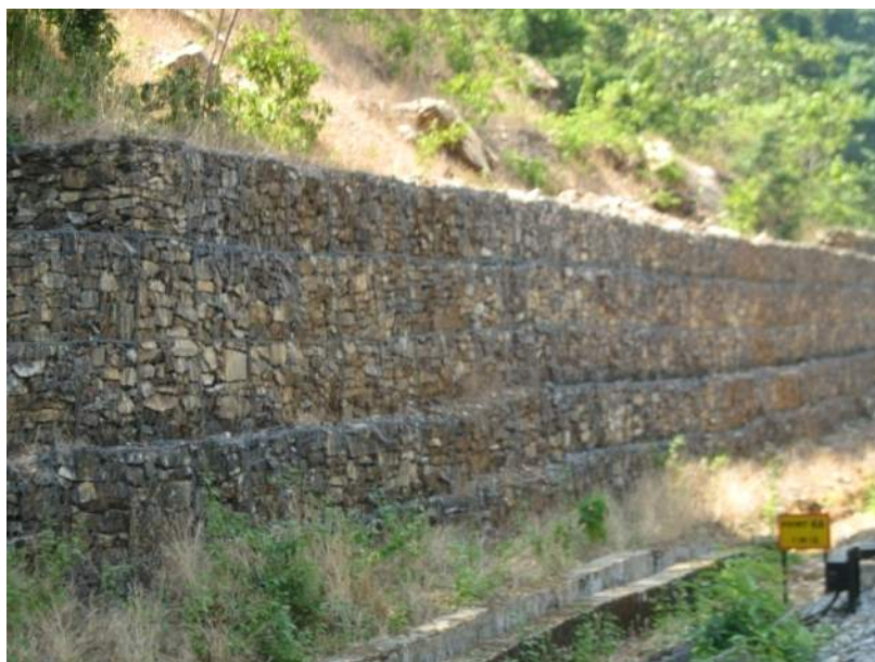
A View of the Gabion structure after station 2 for a stability of weak formation
