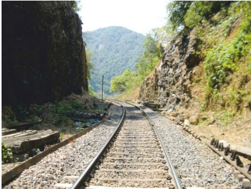
View of cutting in Diorite formation on both sides after Tunnel No. 4
